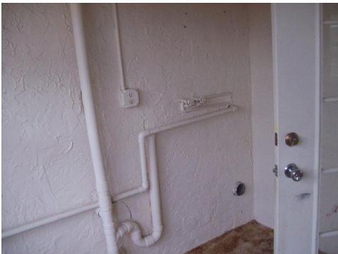
58. Missing Washer And Dryer
