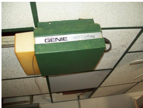
71. Garage Door Opener
