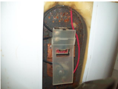
82. Water Heater Control
